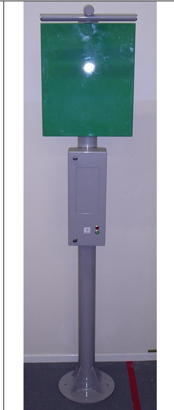
Column Mounted Muster Point
